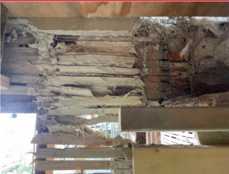
TIMBER LINTEL ROTTEN
