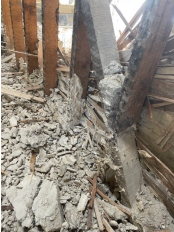
FLAT 7 EXTENT OF ROT CONTINUED ALL THROUGH WALL LHS
