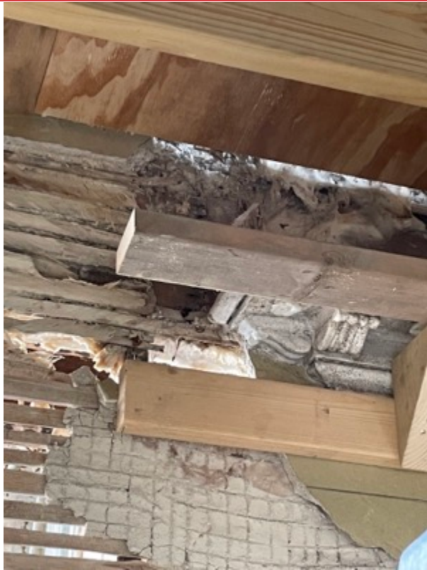
RENDER REMOVED EXPOSES ROT BEHIND CORNICE
